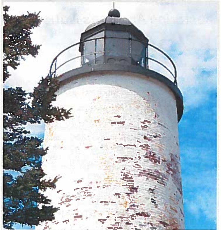
Photo (above): Buildings in Acadia have more than $9 million in deferred maintenance. (NPS Photo. Lighthouse on Baker Island, Acadia National Park).
