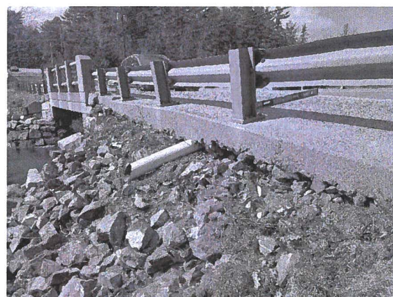
Erosion at Existing Sidewalk Ramp
