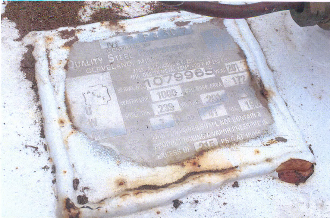
Figure 13. 1000 Gallon Propane Storage Tank (LPG)
