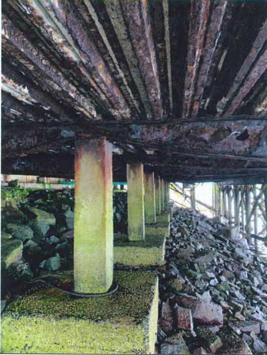
WHARF STRUCTURAL MEMBER DAMAGE
