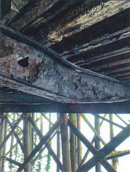
WHARF STRUCTURAL MEMBER DAMAGE
