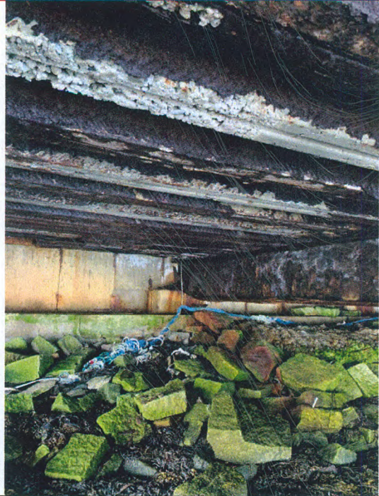
CORROSION TO MEMBERS AND REBAR
