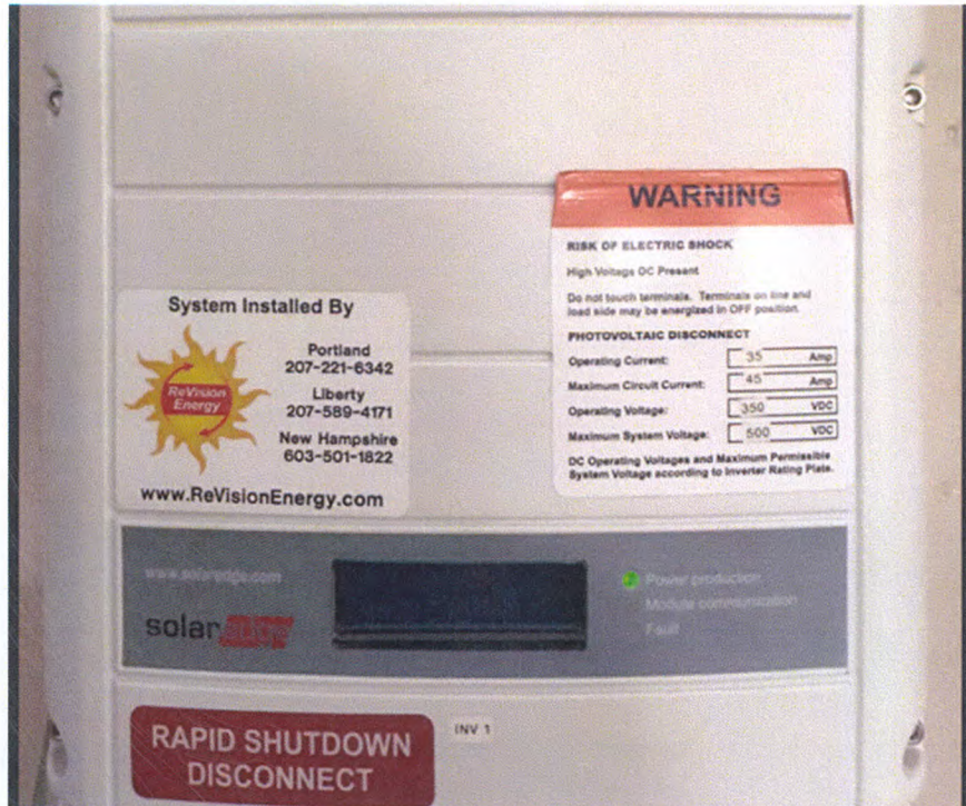
Figure 11. Close up of SolarEdge Inverter Front
