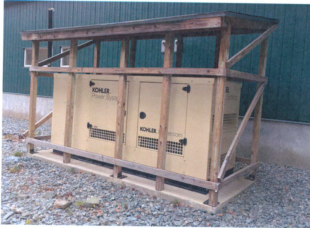
Figure 18. 100 kW Emergency Generator With In-Base Fuel Oil Tank
