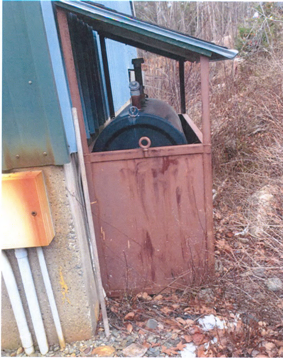
Figure 17. Bus Garage Building 275 Gallon Fuel Oil Tank
