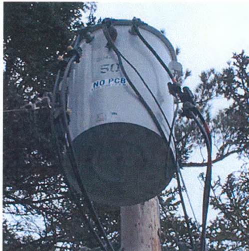
Figure 6. 150 kVA - 240/120 V Service Entrance Transformer
