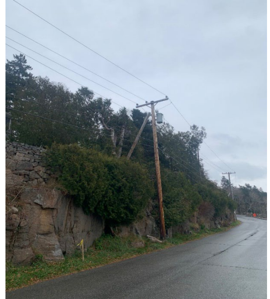
Pole to be removed in Fore ground
