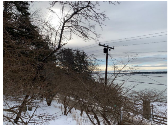
Transformer and pole at Stone South line to remain
