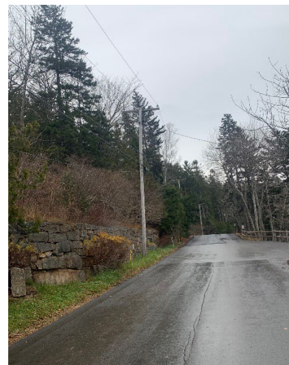
Pole to be Riser Pole and remain Service to Yacht club remain
