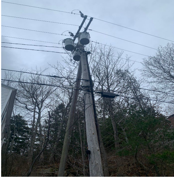
Existing Pole at Matheson Library Line to remain
